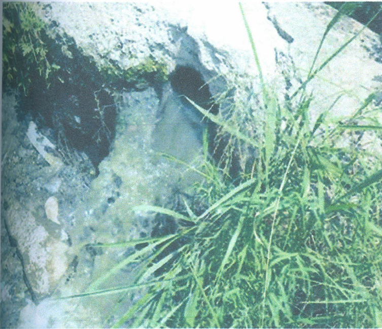
Plate 6: Raw sewer flowing into the environment from the main sewer line. Source: Field Data.
