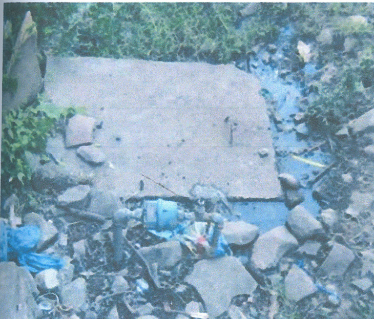
Plate 4: Over flowing manhole from a house around Car Wash area in Lower Migosi. Source: Field Data.
