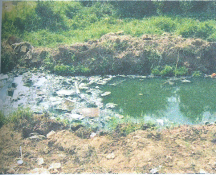
Plate 5: Drainage system filled with raw sewerage and solid wastes in Migosi (Car Wash area) Source: Field Data.
