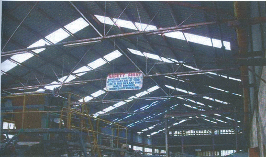
Plate 3: Roof sky lighting system of Highlands Paper Mills Ltd Source: Field survey, 2010
