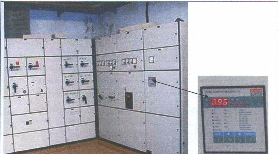
Plate 6: Power control chambers of New KCC Ltd plant with a capacitor bank showing power factor readings of 0.96
