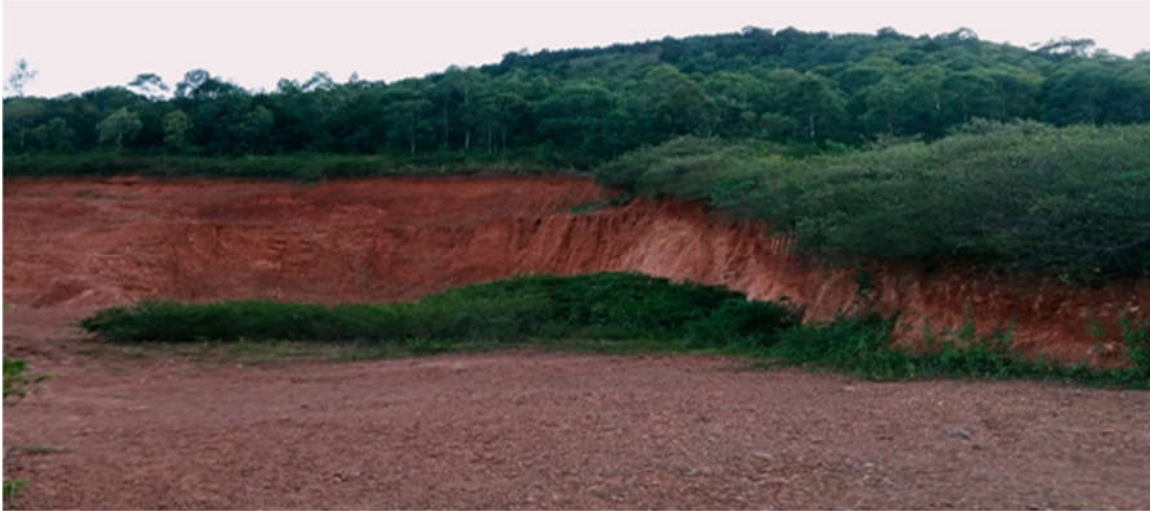
Plate 2: Marram Excavated Land at Wire Hills for Construction of Rural Access Roads and Oyugis Kendu Bay Road.
